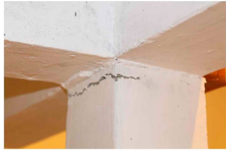
Cracks in Top Ends of Columns on First Storey
