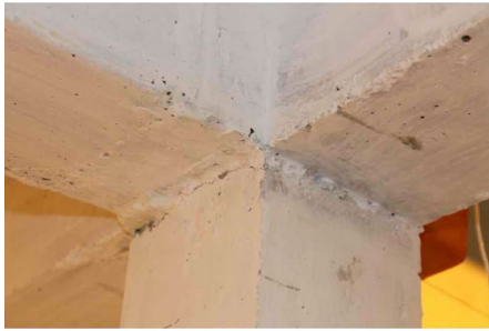
Flexure Cracks in Beam and Column on Ground Storey
