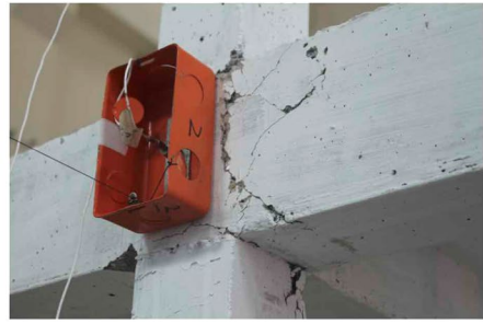
Severe Damage to Joint Panel on Ground Storey
