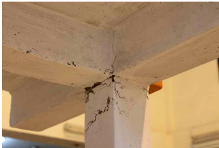
Concrete Crushing at Column Top Ends, Ground Storey
