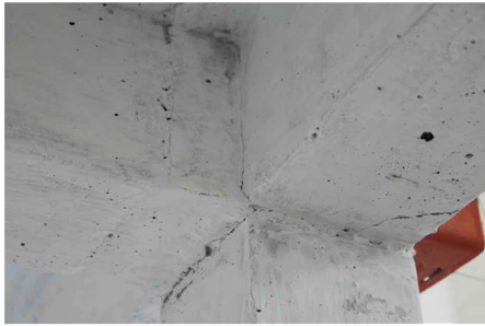
Flexure Cracks in Beams and Columns, Ground Storey
