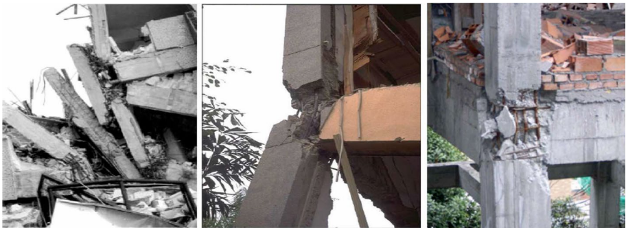
Fig. 1 Joint damageability and, consequent, collapse of structures: from left to right: 1999 Izmit earthquake in Turkey, 1999 Chi-Chi earthquake in Taiwan and 1994 Northridge earthquake in USA (Sharma 2013)
