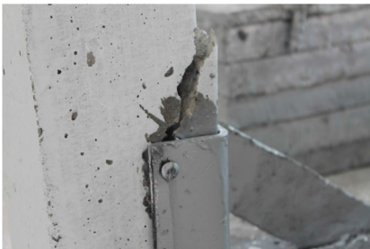
Detachment of haunch under extreme shaking
