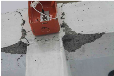
Cover Detachment and Damage in Joint on First Storey
