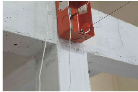
Slight Cracks in Joint Panel on Ground Storey
