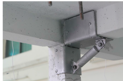
Joint cracks/connection opening under extreme shaking
