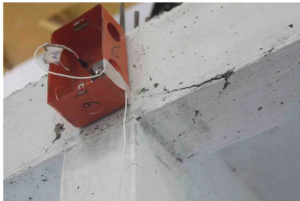
Severe Bat-Like Cracks in Joints on First Storey
