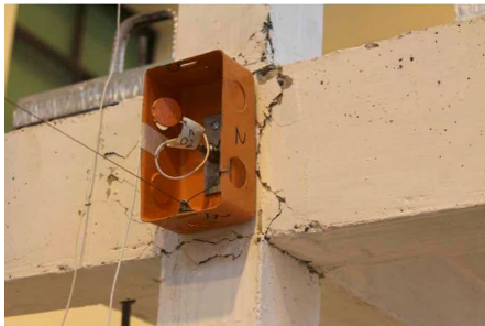
Extend of Damage to Joints on Ground Storey
