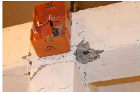
Extend of Damage to Joints on First Storey
