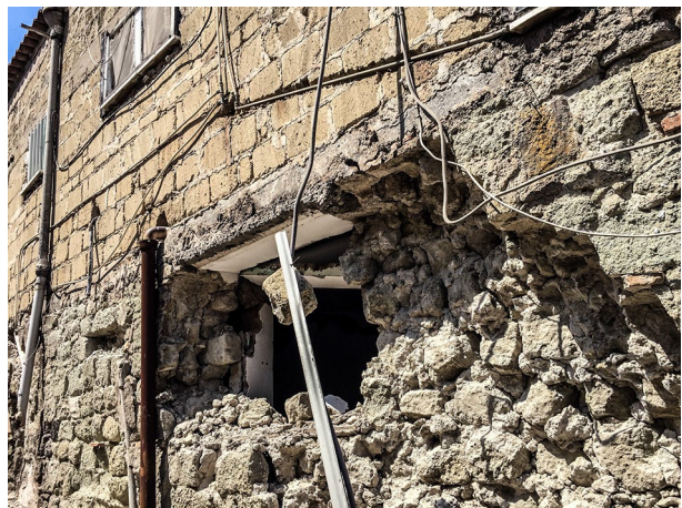
Fig. 23 Failure of the outer wythe of wall: via Epomeo (Lat: 40.742–Lon: 13.9006)
