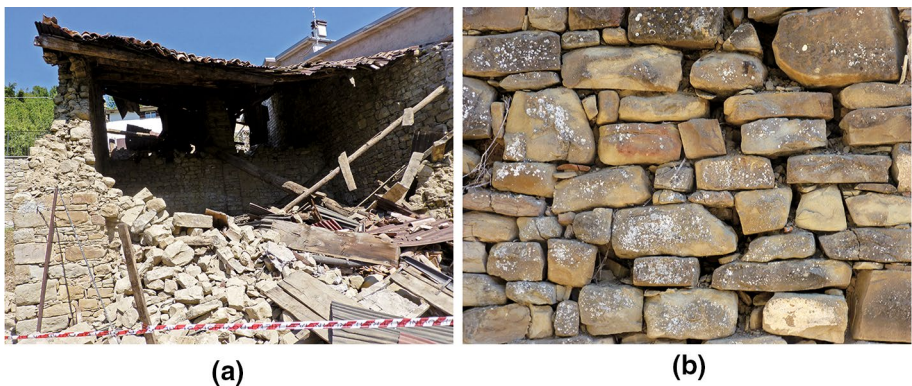
Fig. 12 Masonry disintegration due to poor quality mortar in a reasonably accurate units' assemblage of the external leaf. Amatrice, Cossito: a front view; b detail of masonry on the left-lateral wall
