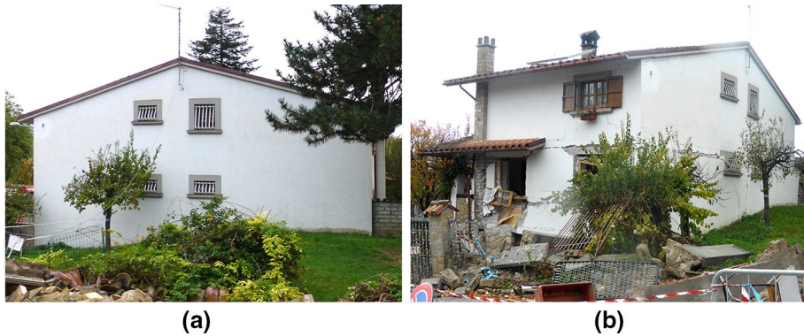
Fig. 21 Solid concrete block masonry building. a After the 24th August event; b after the 30th October event. Amatrice, viale Saturnino Muzii
