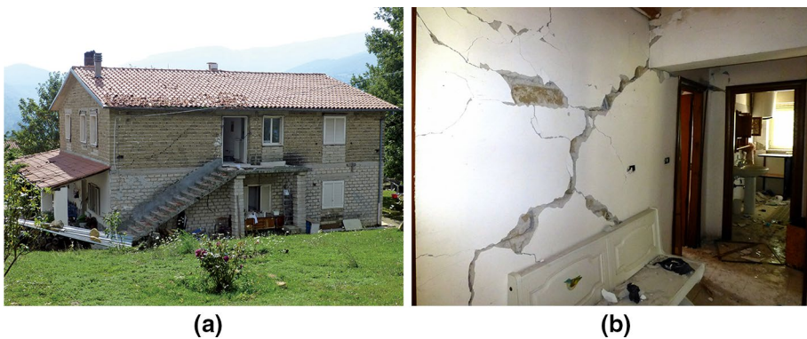
Fig. 22 Solid concrete block masonry (ground floor) and tuff masonry (first floor) building. a External view; b internal view at first floor above ground. Accumoli, Illica
