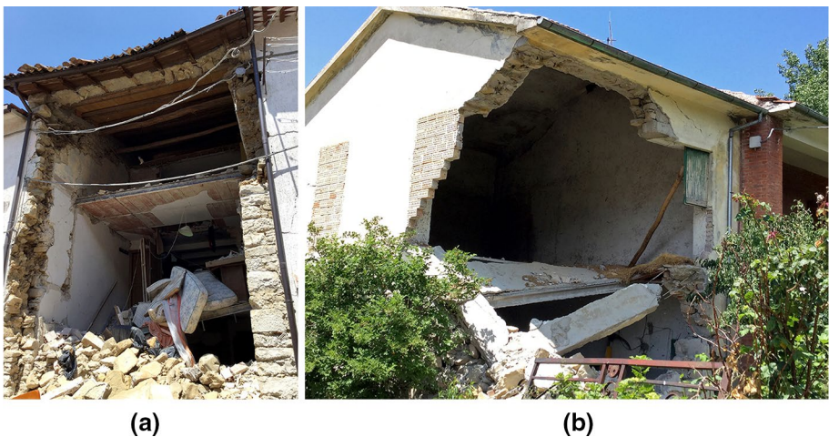
Fig. 6 a I-beam and hollow clay block floor, Amatrice, Retrosi; b Precast reinforced concrete beams and hollow clay block floor, Amatrice, Moletano
