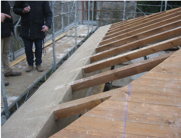
Fig. 8 View of the thick lime mortar layer, pre-consolidating the top portion of the peripheral walls
