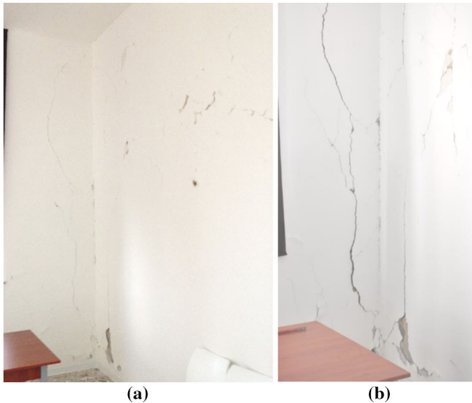
Fig. 16 Damage at the South corner of the building (inside): situation after the Mw6.0 event (a) and after the Mw5.9 and 6.5 events (b)
