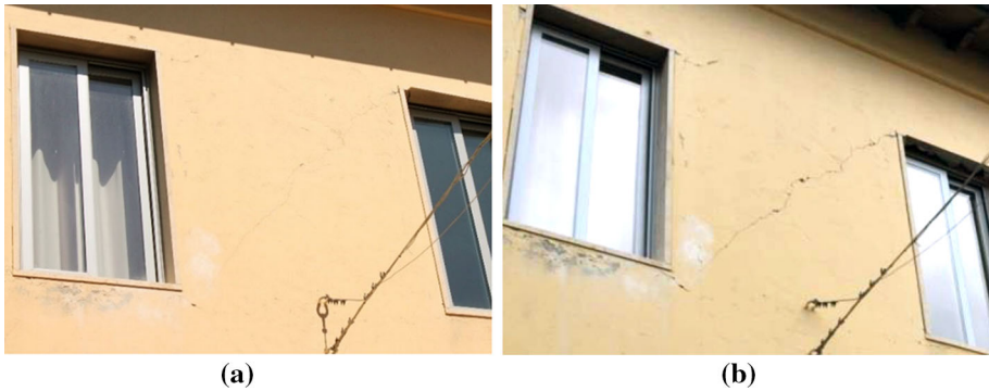
Fig. 11 Shear crack in a second floor pier: situation after Mw6.0 event (a) and after Mw5.9 and 6.5 events (b)
