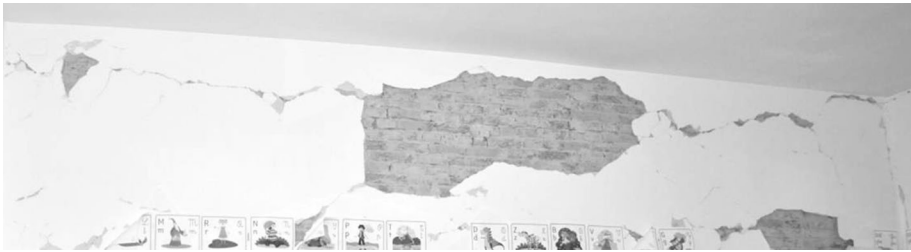
Fig. 12 Damage on 24-cm-thick wall after Mw5.9 and 6.5 events
