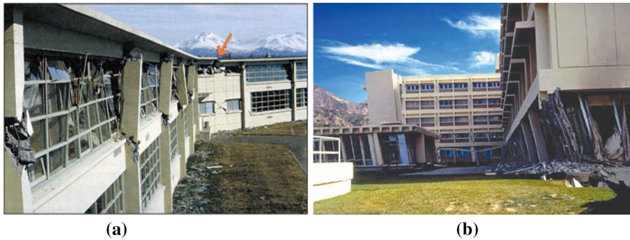
Fig. 1 Earthquake induced damage of L-shape building due to high shear stresses combined with a stress concentration. a Anchorage high school in the 1964 Alaska earthquake, b olive view hospital in 1971 San Fernando earthquake
