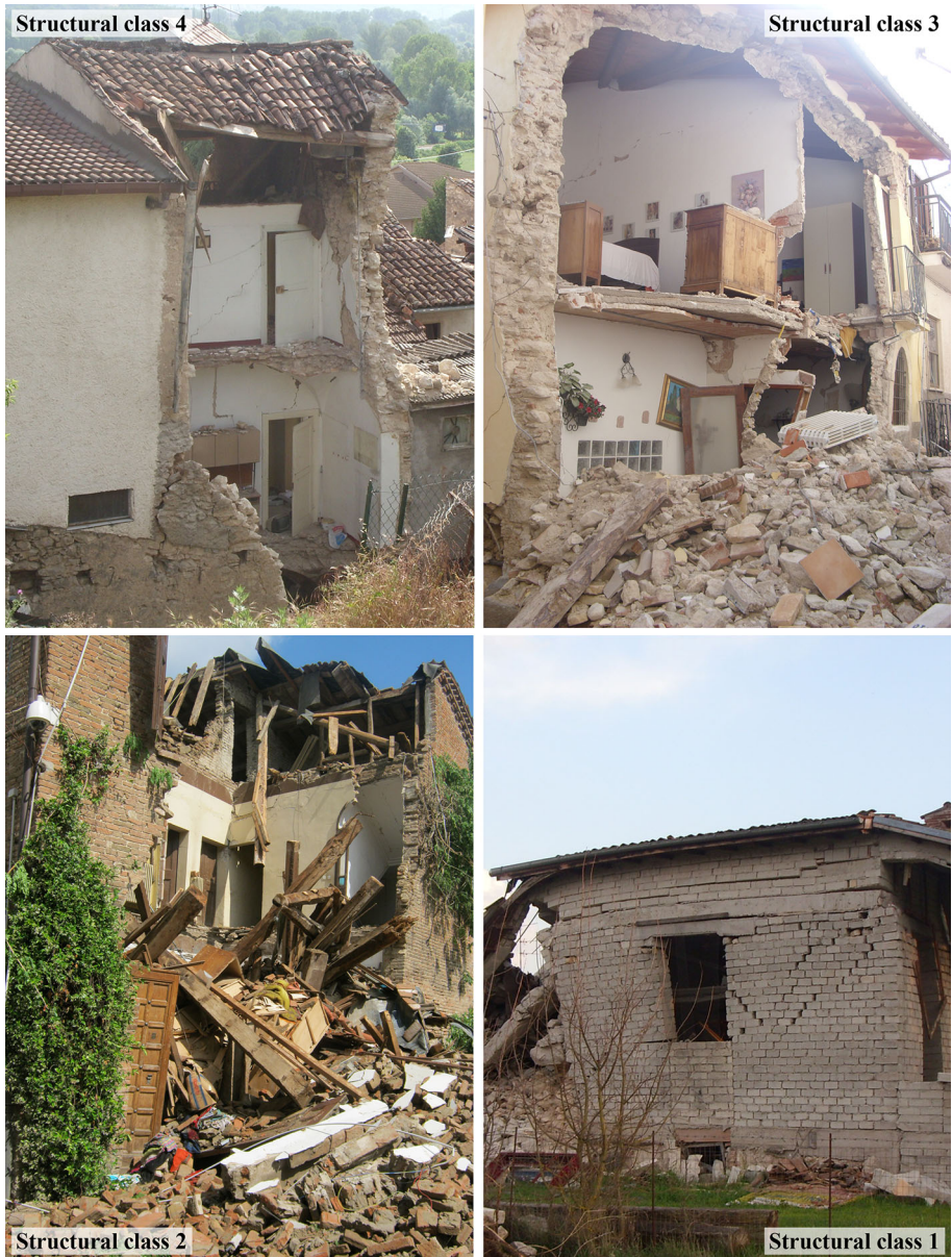
Fig. 10 Examples of earthquake-damaged buildings belonging to the proposed four structural classes: 4 poor quality masonry and flexible slab, 3 poor quality masonry and rigid slab, 2 good quality masonry and flexible slab, 1 good quality masonry and rigid slab
