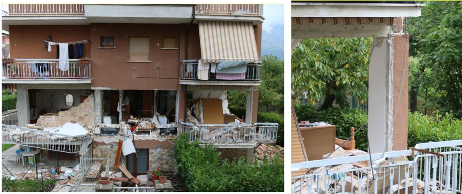
Fig. 7 Partial collapse of the masonry infills of the second level (left) and moderate damage to a beam-column joint (right)
