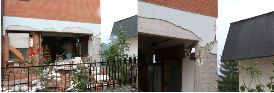
Fig. 9 Damage to the brick masonry infill (left) and details of the column damage (right)
