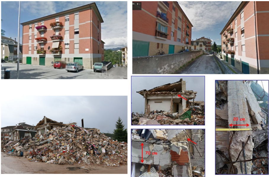
Fig. 6 Images of two collapsed RC buildings before (top) and after (bottom, on the left) the August 2016 earthquake, with some details of buildings' characteristics and damage (bottom, on the right)
