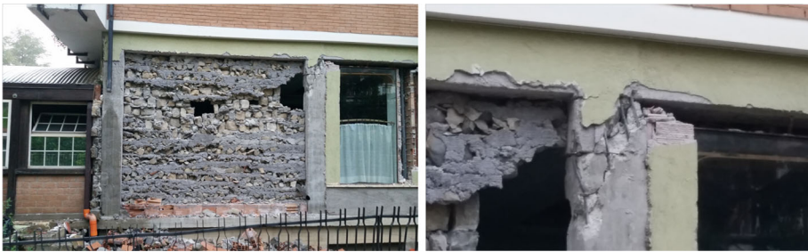
Fig. 10 Damage to the stone masonry infill (left) and details of the column damage (right)
