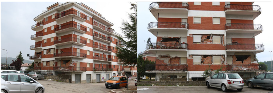
Fig. 8 Partial collapse of infill panels at the second and third storey
