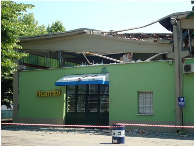
Fig. 1 Structural collapse of a precast building occurred during the Emilia earthquake (May 2012) due to loss of support of the roof beam
