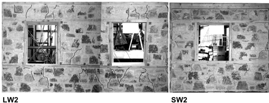
Fig. 19 TLMBM-BS. Observed damage in the walls LW2 and SW2 at the ground floor of the interior of the model after Test 16BS [Kalamata earthquake: 0.42 g(X)/0.37 g(Y), Table 1]
