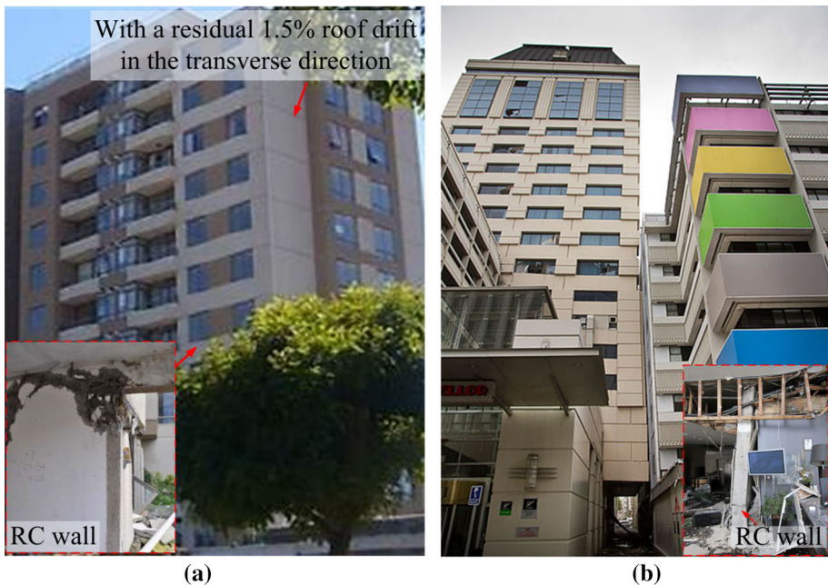
Fig. 1 Observed damage of RC wall after earthquakes: a Plaza del Rio building A, 12-story, demolished after 2010 Maule earthquake (NIST 2014); b hotel grand chancellor, 26-story, demolished after 2011 Christchurch earthquake (Wikipedia 2017)
