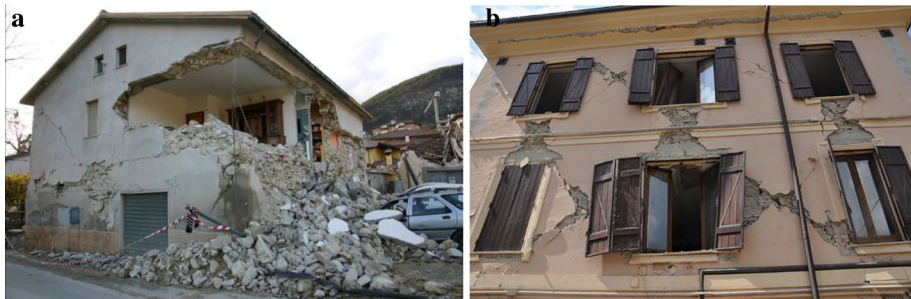
Fig. 1 Stone masonry buildings after the 2009 L’Aquila earthquake that failed due to an out-of-plane mechanism ( a photo: A. Dazio) and an in-plane mechanisms ( b photo: A. Penna)
