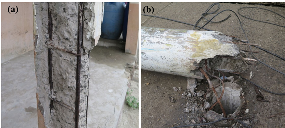
Fig. 9 Damaged column (a) and collapsed electrical post (b)
