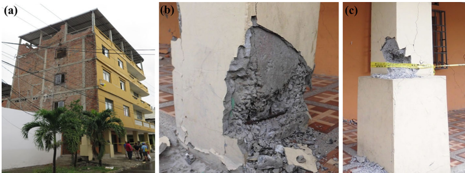
Fig. 6 5-Storey RC building with masonry infills located in Tarqui (Manta) (a), and its damage to the ground-floor-columns (b, c)
