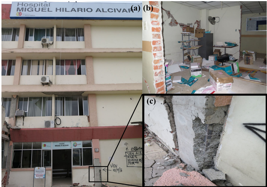
Fig. 13 a Damage to the retrofitted Miguel Hilario Alcivar hospital in Bahía de Caráquez, b interior damage to partitions and content, and c structural damage in the wall boundary
