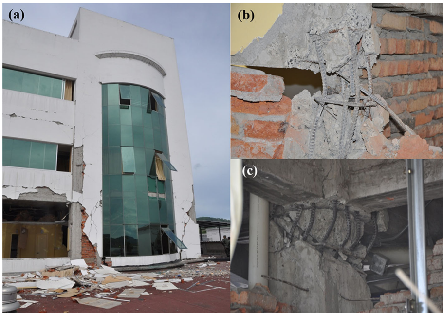
Fig. 14 a Damage to the building tower of the Solca hospital in Portoviejo, b failure of a non-structural column, and c shear failure of an interior column
