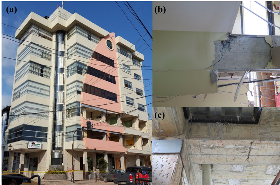
Fig. 10 7-storey Hotel Ceibo Dorado in Portoviejo overall damage (a), damage to the staircase (b) and perimetral beams (c)
