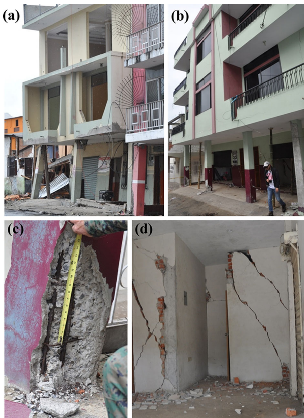
Fig. 7 Soft-storey buildings in Manta (a), damage to the columns (c) and partitions (d)
