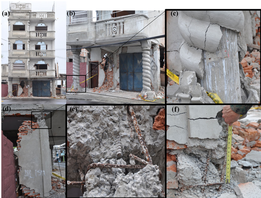
Fig. 8 4-storey RC building with several deficiencies located in Manta (a), structural irregularities and heavy cladding (b, c), and detailing deficiencies (d, e, f)
