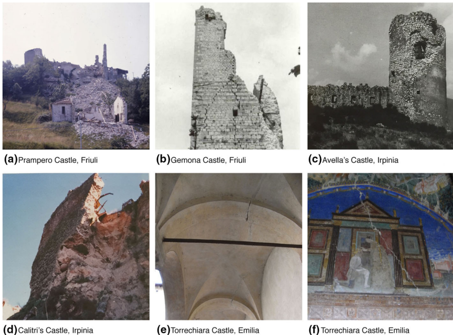
Fig. 6 Typical castles hit by the earthquakes in Friuli (a, b), Irpinia (c, d) and Emilia 2008 (e, f)
