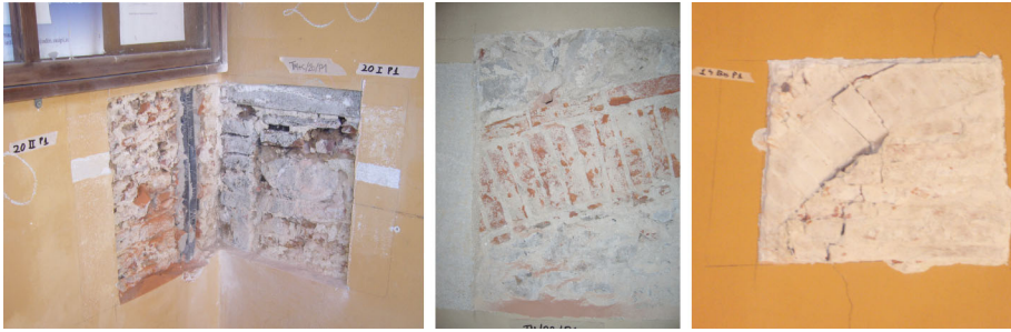
Fig. 13 Discontinuities of vertical masonry walls: absence of connection between perpendicular walls, arches identified in correspondence of the first floor level, probably old windows currently closed
