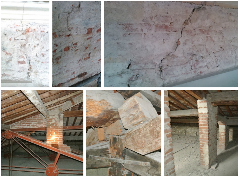
Fig. 18 Degradation and problems affecting the roof structure of the Palace
