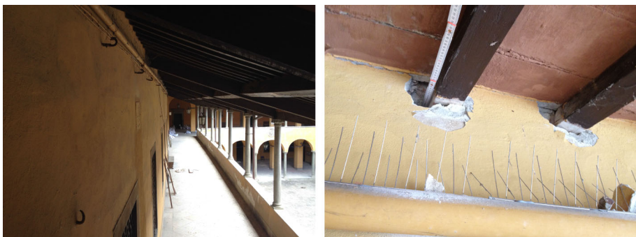
Fig. 16 Internal colonnade (1st floor): relative displacements between wooden elements and masonry walls
