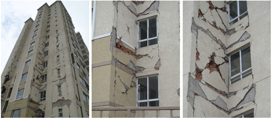
Fig. 10 Diagonal cracking of the IM walls in a 16 storey high-rise building façade
