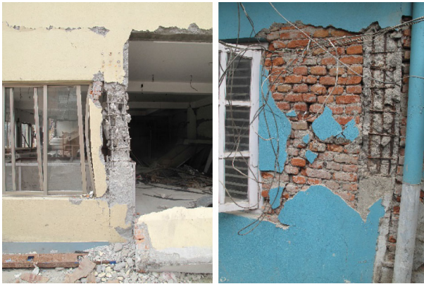
Fig. 15 RC buildings subjected to short-column mechanism
