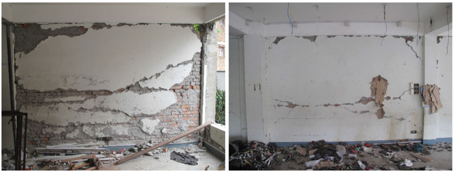
Fig. 11 Shear friction failure observed in interior partition walls of low and medium-rise residential buildings
