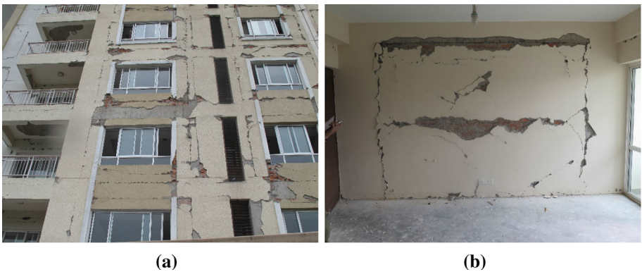
Fig. 9 Detachment of the IM panel from the surrounding RC structural elements by the a Exterior IM walls from a 16 storey building façade, and b Interior partition wall
