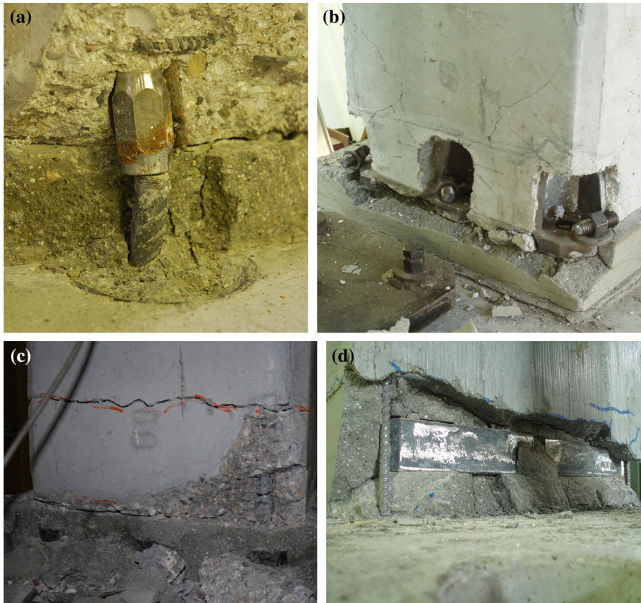
Fig. 10 Failure modes: a post-screwed protruding bars, b standard sockets, c overturned sockets, d couplers (failure not attained)
