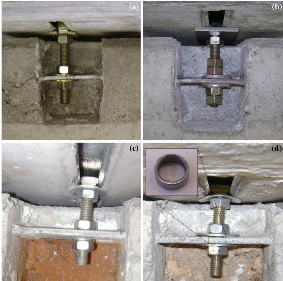
Fig. 4 Panel column subassembly (PCS) top connection details. a PCS A, b PCS B, c PCS C and d PCS D
