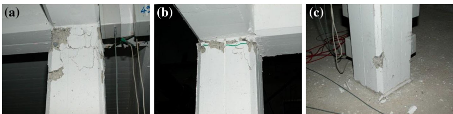
Fig. 4 Visible damage in the specimen after the 0.20 PGA test: a extensive spalling at the top of columns (C3); b light spalling and flexural cracking at the top of corner columns (C1); c base of column C3
