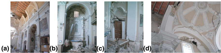
Fig. 14 Collapse mechanisms detected by Y direction pushover analysis: a arches in the nave, b–c walls and buttresses in lateral chapels, d transept arches
