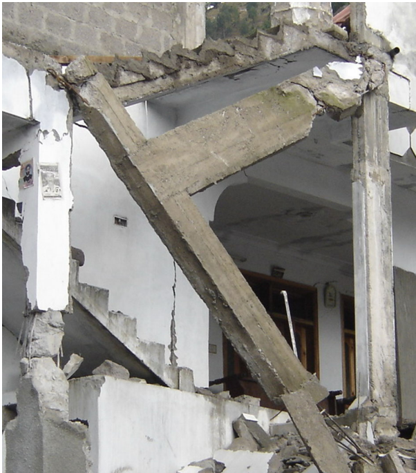
Fig. 4 Damage of typical non-engineered structure after Kashmir earthquake (2005)
