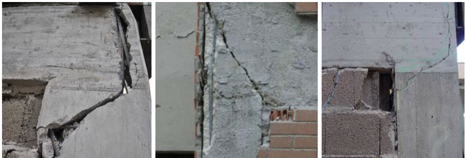
Fig. 2 Local shear failure of frame due to interaction with infills under seismic loads
