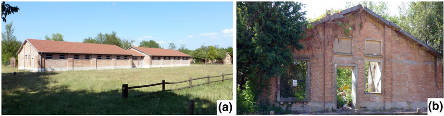
Fig. 25 Campo di Fossoli— a restored barrack used as visitor and exhibition centre; b damaged barrack
