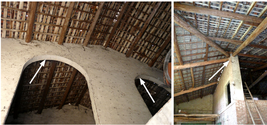
Fig. 9 Different structures of the roof in the haylofts—arrows indicate damage
