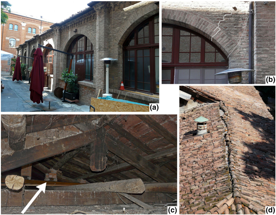
Fig. 22 The Mattatoio — a lateral view; b cracking of the arch opening; c critical situations on roof truss; d roof tiles displacement
