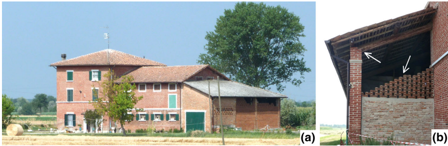
Fig. 8 a a typical rural house in Reggiolo; b the portico with collapsed hollow brick wall and cracked masonry pillar
