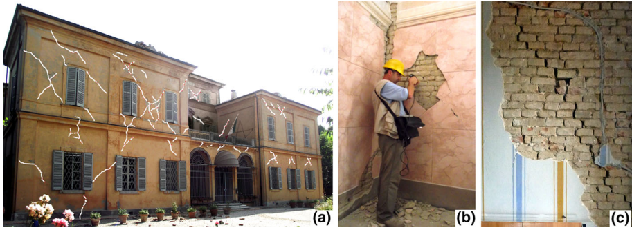
Fig. 6 Retirement home—a external view; b PNT-G tests; c crack pattern
