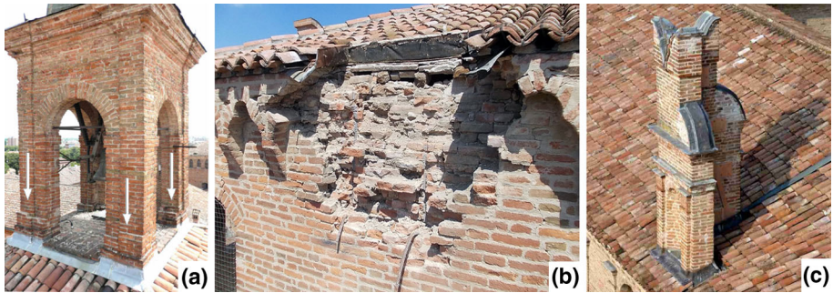
Fig. 18 Palazzo dei Pio — a bell tower atop the Torre dell’Orologio b collapsed merlon on the Torre del Passerino c consolidated merlon on the main façade
