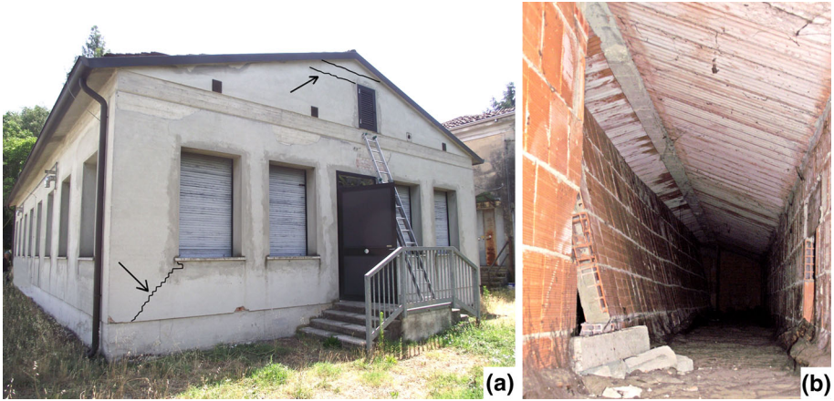
Fig. 10 Social Centre— a external view; b overturning of the upper masonry roof walls
