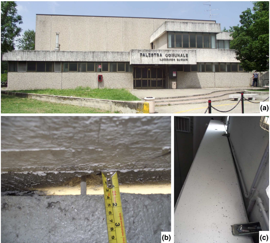
Fig. 11 Magnani sports hall— a general view; b , c details of the connections of the panels
