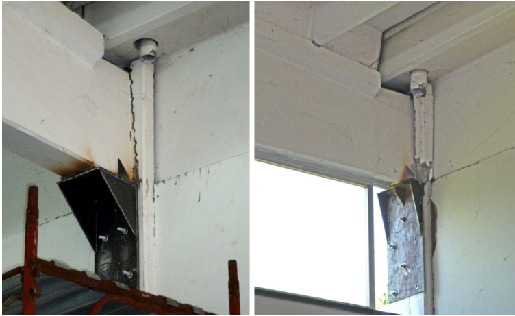
Fig. 12 Textile factory in Reggiolo: reinforcement added to the support of a precast beam after the earthquake
