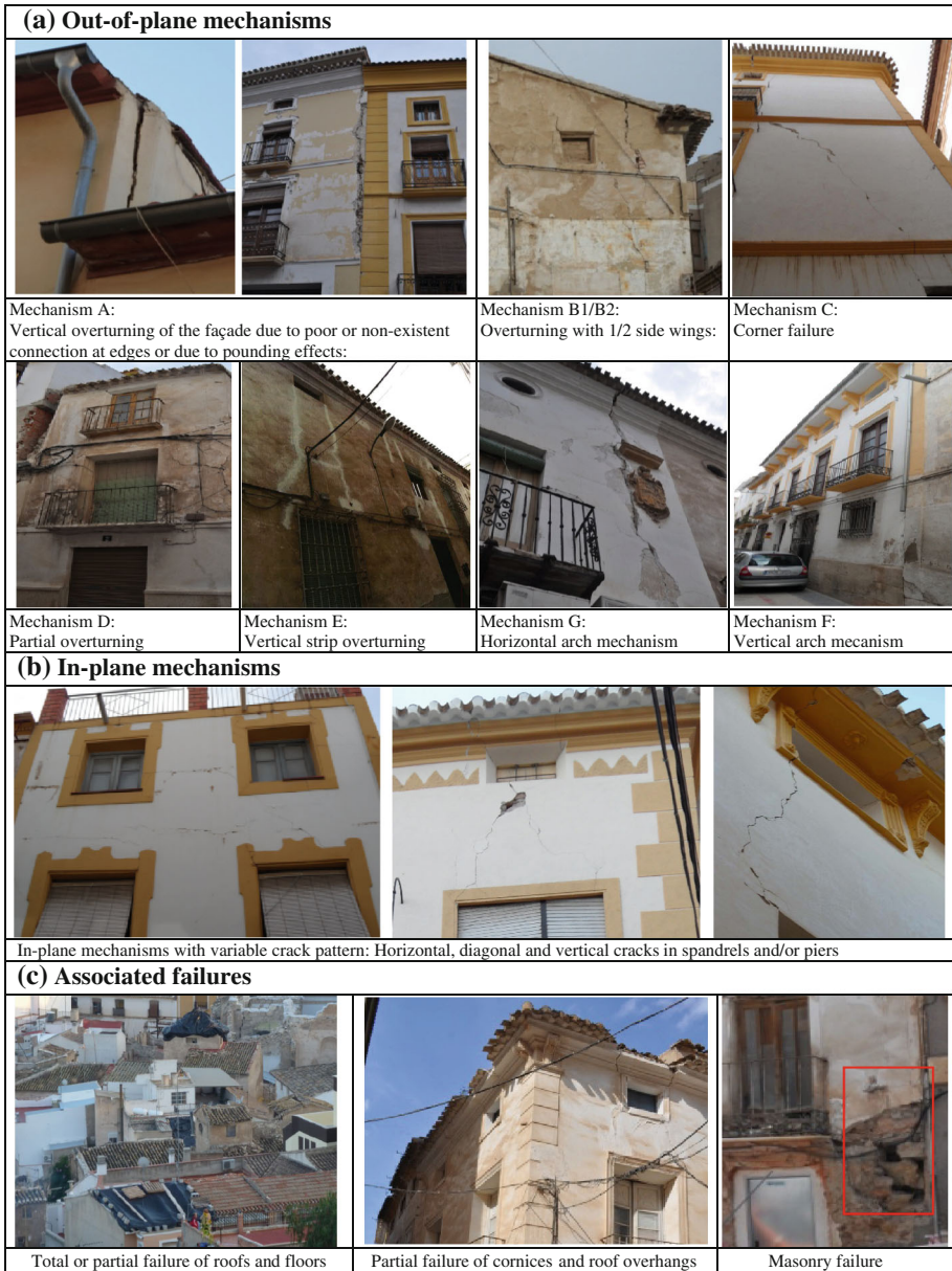
Fig. 12 Collapse mechanisms observed in the surveyed area: a out-of-plane mechanisms, b in-plane mechanisms and c associated failures
