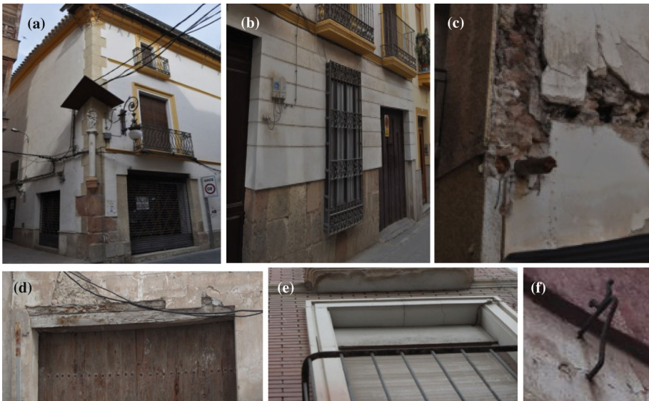
Fig. 9 Reinforcement elements: a quoins, b plinths, c floor and wall timber ties or timber ring beams, d timber lintels, e stone frames around openings and f iron ties
