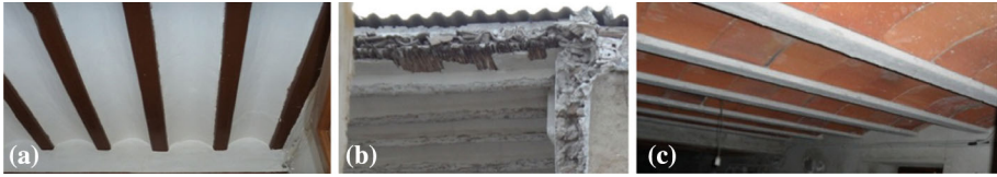
Fig. 7 Horizontal structures: a timber floors (timber beams and joists with lightweight masonry vaults), b roofs (reed and plaster deck, “cañizo”, under ceramic curved tiles) and c new RC floors (RC beams and joists with ceramic vaults)
