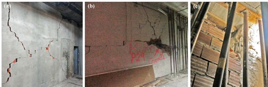
Fig. 11 In-plane failures in masonry infill panels: shear diagonal cracking (a), horizontal sliding (b), corner crushing and induced brittle failure of RC column (c) ( Calconsa 2011 )
