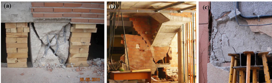
Fig. 9 Brittle failure of “squat” column (a) ( Vidal et al. 2011 ), masonry staircase (b) , beam-column joint (c)
