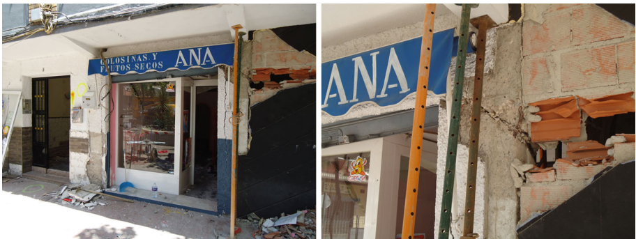
Fig. 19 Example of a shear-damaged column due to the failure of the adjacent infill panel
