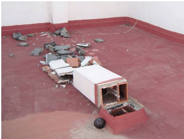
Fig. 6 Collapsed chimney on a flat roof
