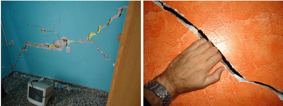
Fig. 11 Examples of damaged partition walls during the Lorca earthquake
