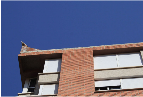
Fig. 2 Building with a partially collapsed parapet wall
