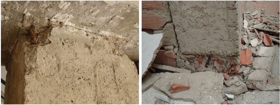
Fig. 17 Examples of failure at the construction joint of a beam–column connections
