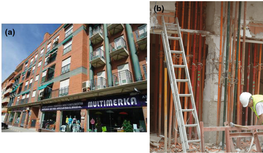
Fig. 7 a Buildings with a soft-storey, b severely damaged column
