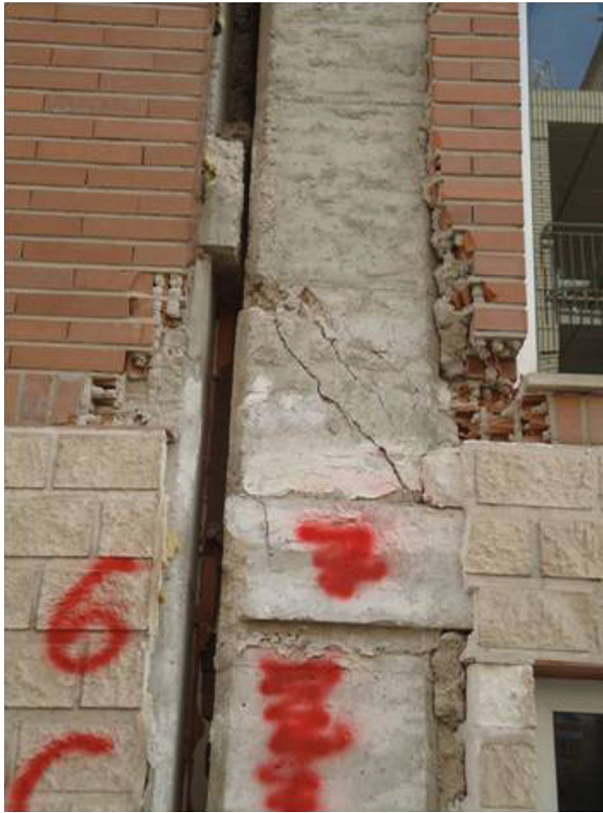
Fig. 13 Example of buildings that suffered damage due to pounding effects
