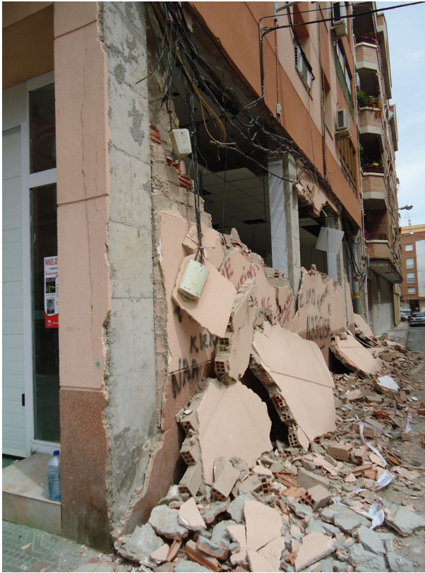
Fig. 3 Damaged masonry infill walls at ground floor
