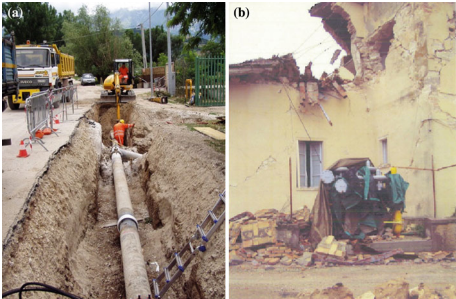
Fig. 4 Damage to stations: a repairs to the input/output network of Onna M/R and inclusion of stop-system; b RG housed in a masonry kiosk closed to building and damaged following the 6 April 2009 earthquake (photos courtesy of ENEL Rete Gas)
