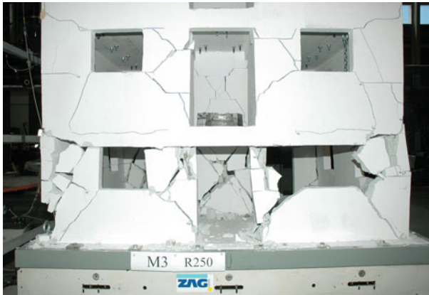
Fig. 23 Damage to the walls in the ground floor of model M3 at ultimate state
