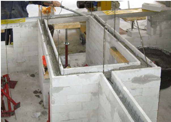
Fig. 11 Concreting the bond-beams above internal walls. Reinforcement of bond-beams and tie-columns can be also seen
