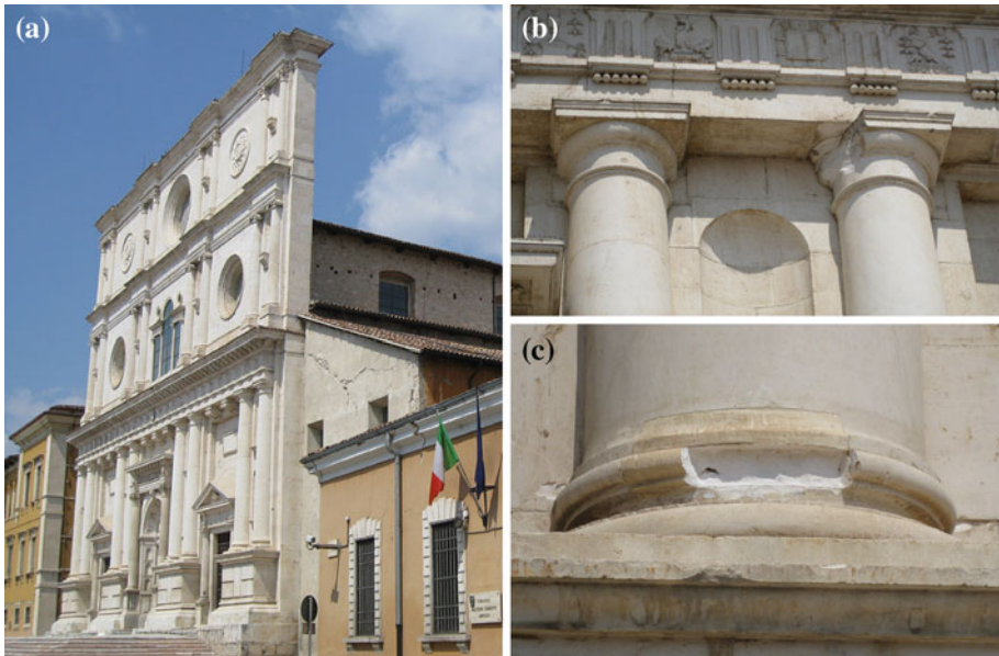
Fig. 9 S. Bernardino basilica in L'Aquila: a the façade; b–c details of some local crushing of marble elements due to out-of-plane overturning mechanism
