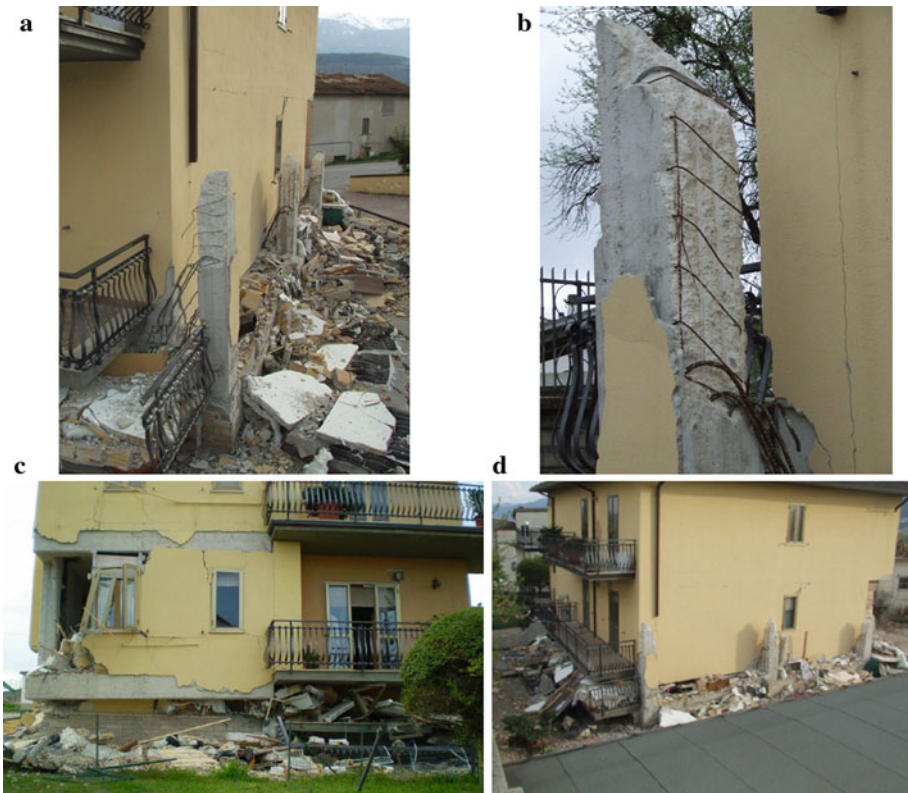
Fig. 4 Storey mechanism: details of the columns on back view (a); structural column details (b); lateral view (East) (c); back view (North) (d)
