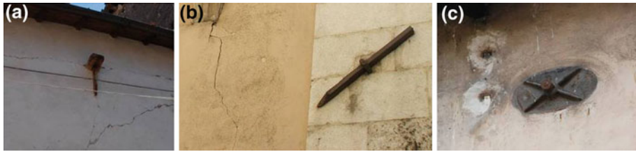
Fig. 8 Traditional reinforcement: a timber tie, b wrought iron cross tie inserted in a quoin and c twentieth century steel tie with end plate
