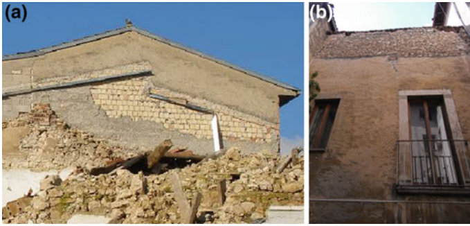
Fig. 3 Example of masonry fabrics with later addition of upper storey and concrete elements
