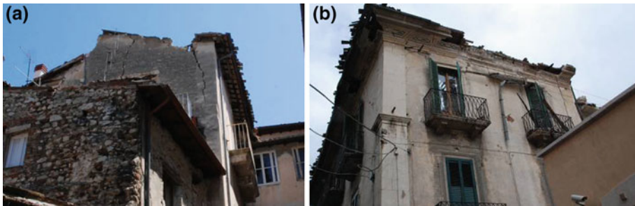
Fig. 14 Collapse of roof structures
