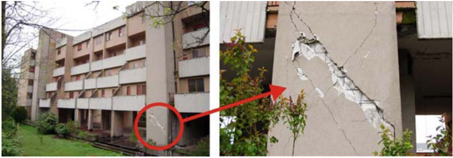
Fig. 1 Failure of a structural wall during the 2009 L'Aquila earthquake. Photographs by M. Rozman and K. Rejec, 2009
