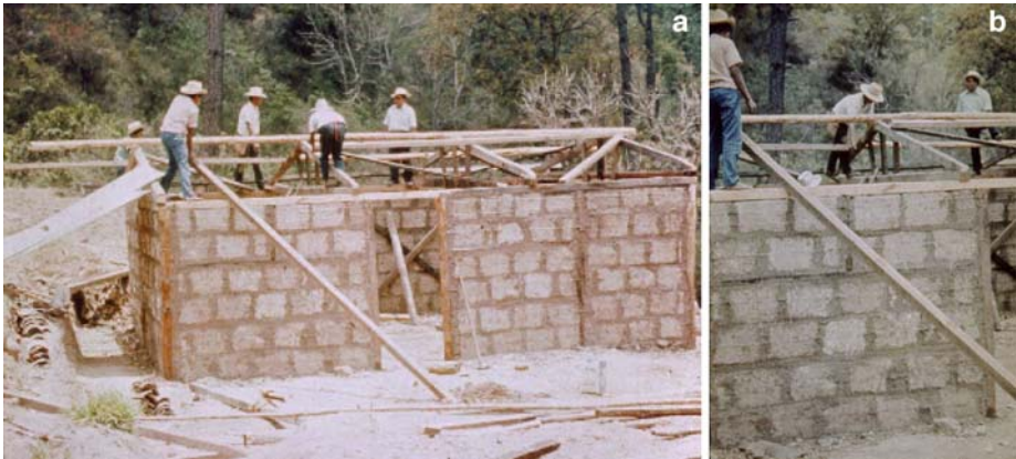
Fig. 59 OXFAM/World Neighbours Rebuilding Programme after the 1976 Guatemala earthquake used a timber frame infilled with locally made concrete blocks (a,b) (Photos from OXFAM Guatemala)
