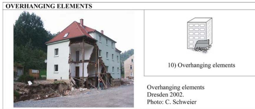
Figure 6. Damage type – Overhanging elements.
