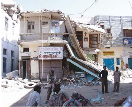
Figure 8. Damage type “Multi layer collapse”; India, 2001. Photo: M. Markus.
