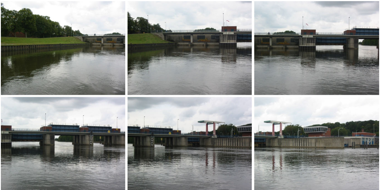
Fig. 22 An overview of the Lesumer Sperrwerk as seen from the river's surface
