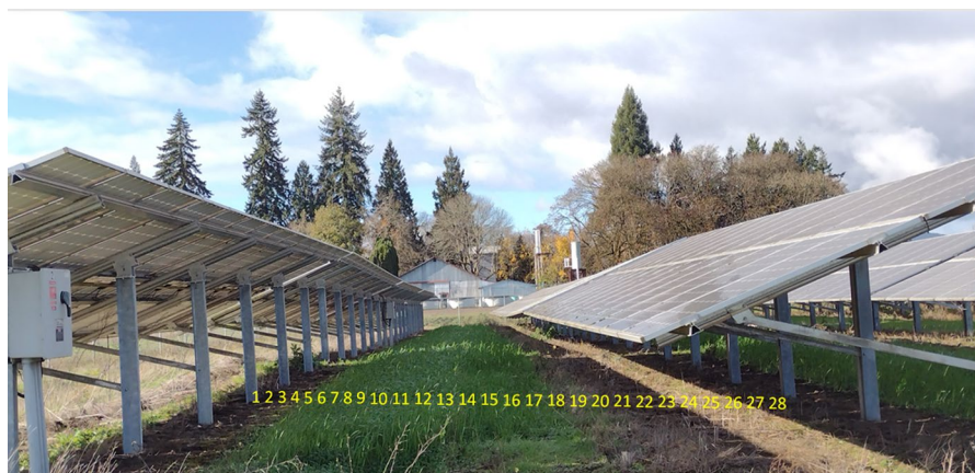
Fig. 2 Transect under photovoltaic panels. The figure shows the 28 measuring points along the transect, between two rows of photovoltaic panels. The points were marked on the ground, to allow measuring exactly in the same place at every measuring time
