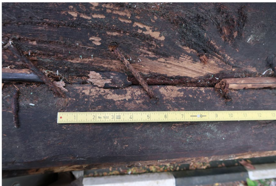
Fig. 20 Example of the method of caulking. Note a heavy deterioration of the caulking coir fiber and battens
