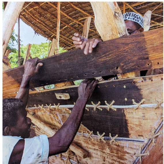
Fig. 8 Method of edge joinery between planks. Note the dark staining caused by heating the planks over the fire to bend them to a desired shape. Modified after the House of Wonders and Zanzibar National Museum of History and Culture (2004)
