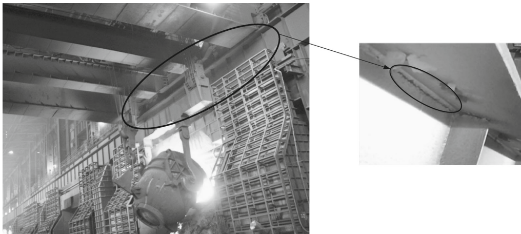
Fig. 9 Fatigue crack being detected at the weld joint between the upper flange and web plate of the steel CRG
