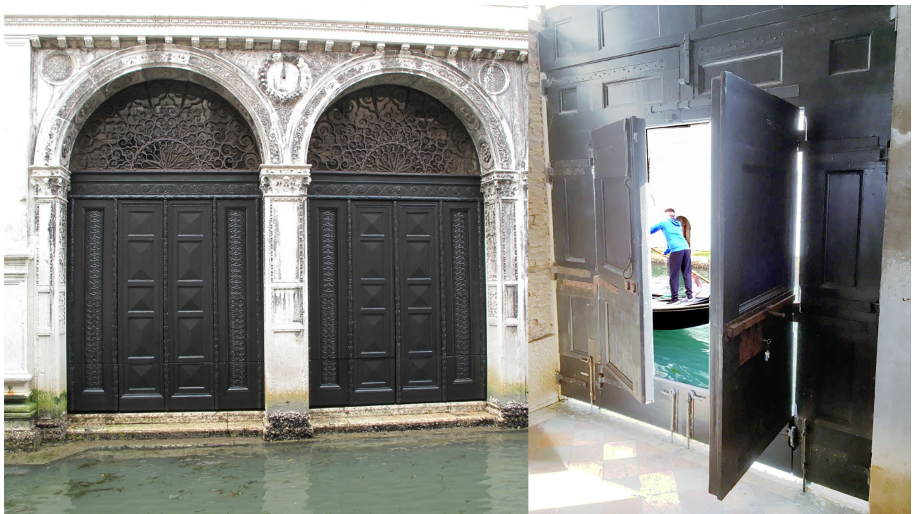
Fig. 15 The water-doors after restoration. The image from the inside shows the separation between the upper and lower parts, facilitating maintenance work
