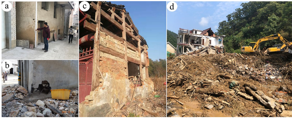
Fig. 8 Buildings affected by the 2019 WZW debris flow across various damage degrees: a slight damage, b moderate damage, c extensive damage, d complete damage
