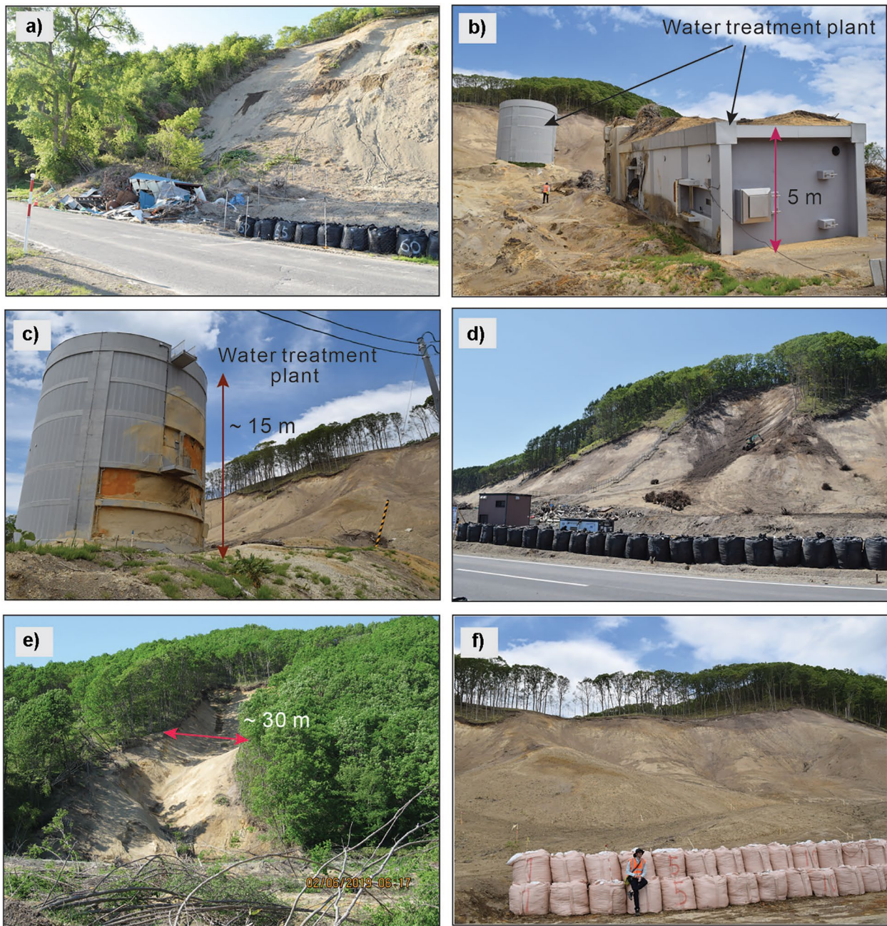
Fig. 5 Field survey photos of landslides following the September 2018 earthquake around the Atsuma area of Hokkaido (Japan). a A shallow landslide near a road. b, c A water treatment plant destroyed
