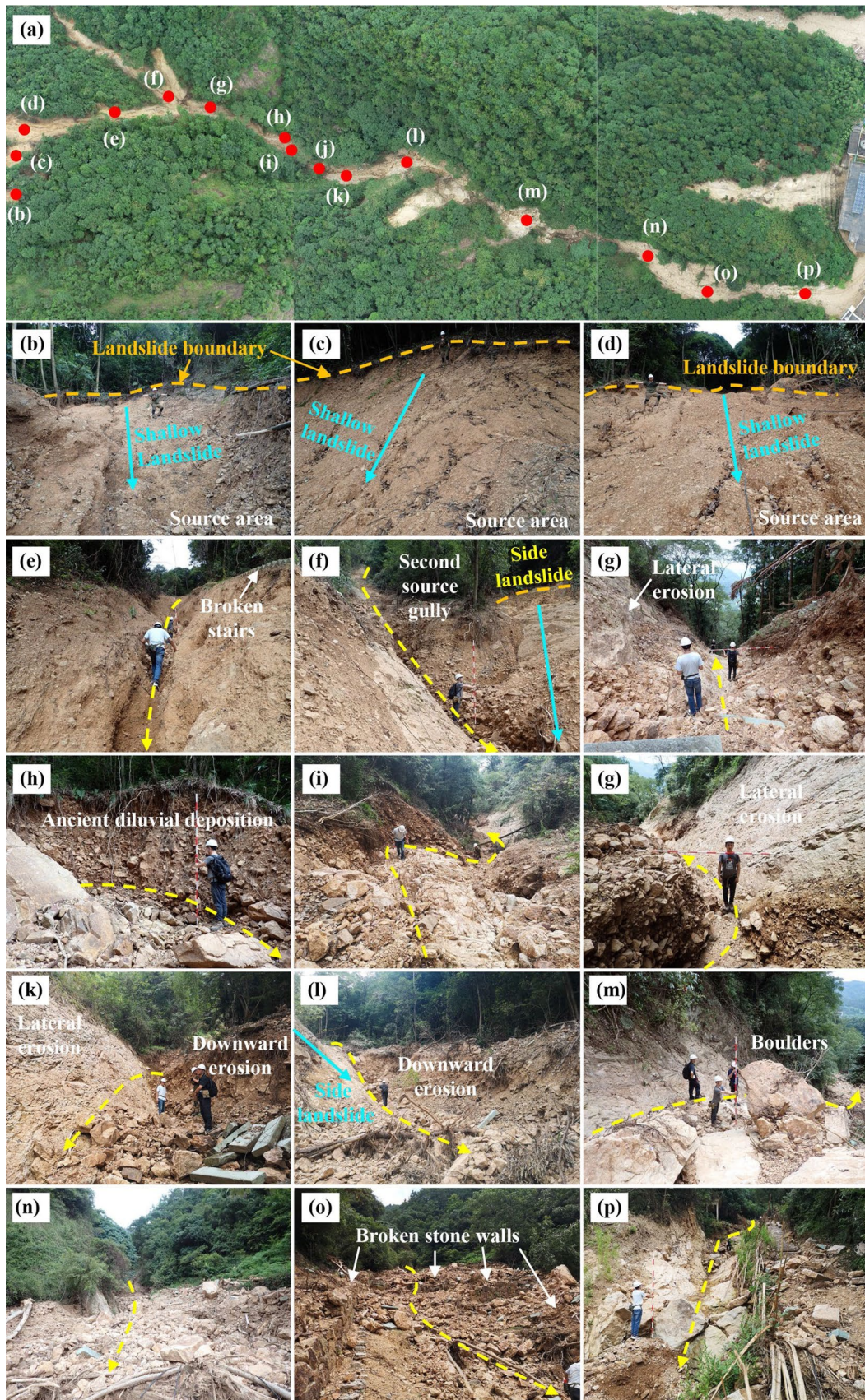
Fig. 17 Photographs describing the DF2 gully from the main source area to the toe. The spliced image (a) illustrates the investigated positions of the detailed features from (b) to (p) along the gully
