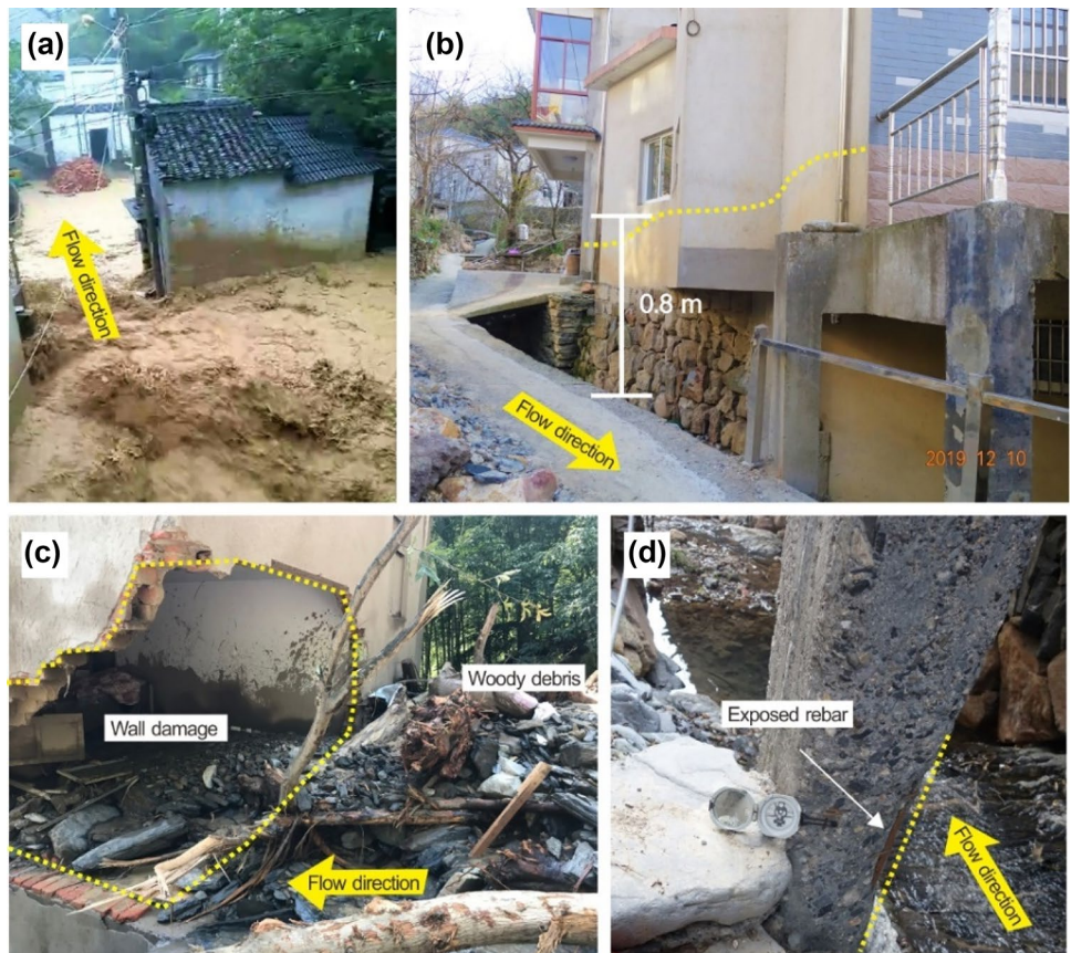
Fig. 11 Field photos in the village that the debris flow passed through. ((a) Screenshot from the video taken by an eyewitness; (b) muddy trace on a building; (c) damaged housing along the pathway of the stream; (d) abrasion of a concrete column)
