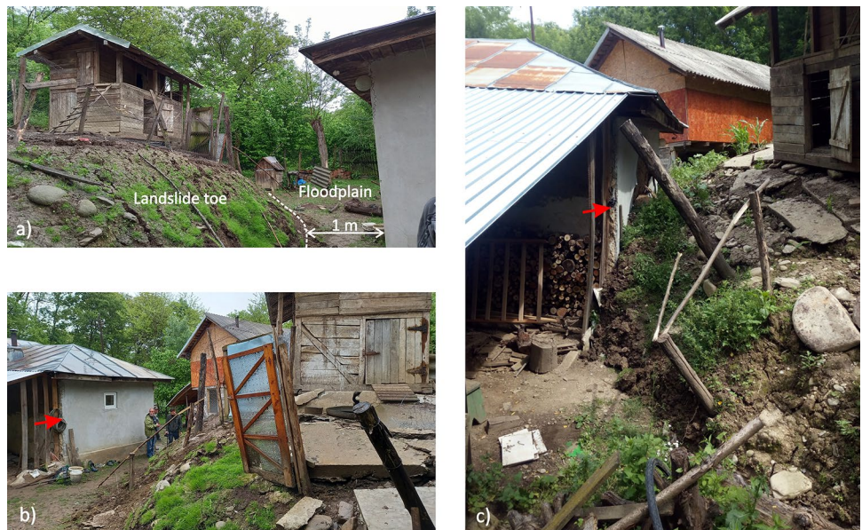
Fig. 12 The landslide toe: (a) view to upslope and (b) view to downslope (photo taken on 25 May 2021); (c) the landslide toe reached the house on 6 July 2021 (photo credit: Daniel Ioniță). The red arrow indicates the same corner of the house
