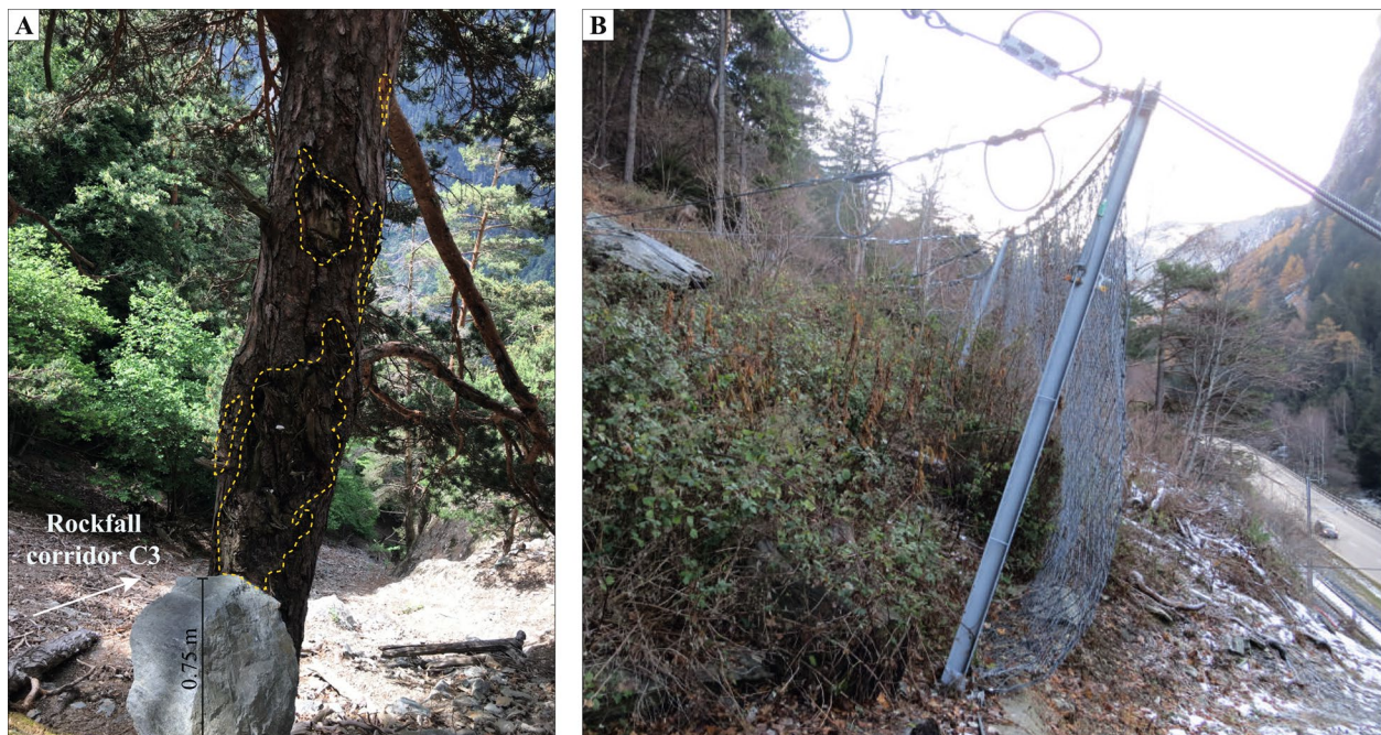
Fig. 3 View of (A) a multi-impacted pine stem (yellow dotted line) sampled at the vicinity of the cliff and (B) rockfall protection barriers installed in the lowest portion of the talus slope
