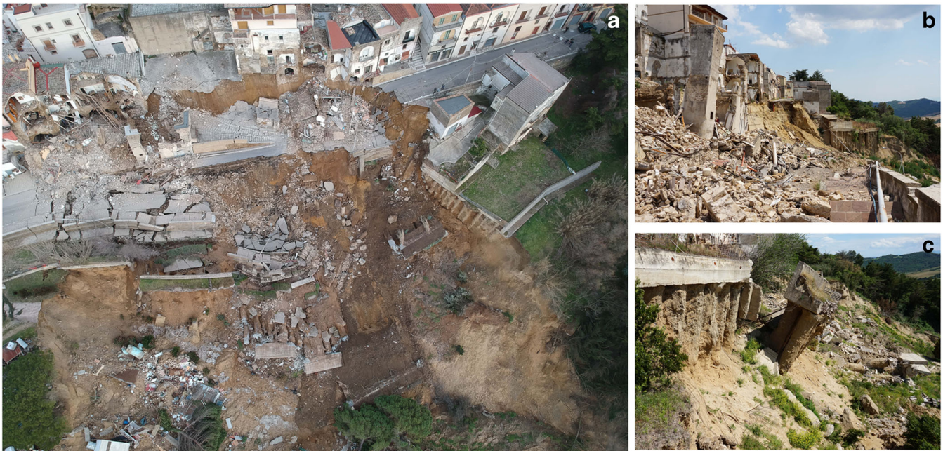
Fig. 2 Upper scarp of the landslide and damages to structures and bulkhead
