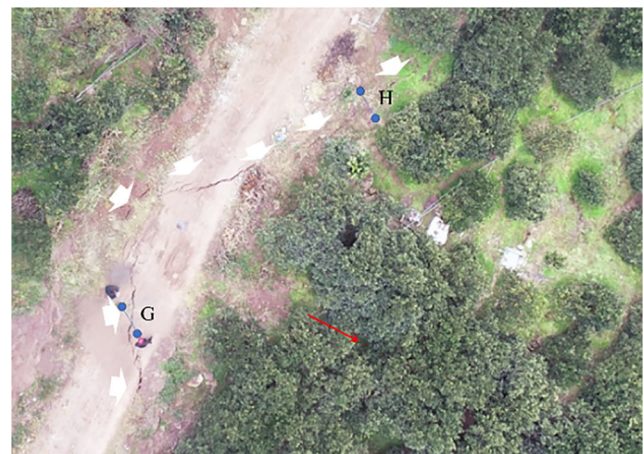
Fig. 18 Retrogressive zone photo. The crack on the left side extends very long, about 15 m, and the crack on the right side is only visible on the road surface. G and H are the measuring points of crack relative displacement
