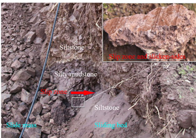
Fig. 14 Photos of slide mass, slip zone, and sliding bed in the trailing edge. Right-upper map is the photo of slip zone, with a large area of polished surface and striated scratches (photo taken by Bolin Huang after failed)
