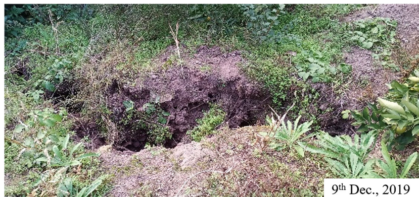
Fig. 6 Photos of transverse cracks in the middle of the slide mass, taken on December 9
