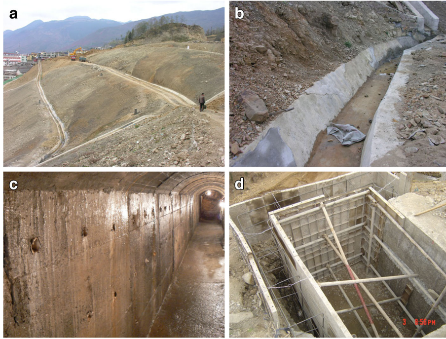
Fig. 4 Treatment projects. (a) Stair shape after reducing load. (b) Drainage channel on the slope surface. (c) Adit inside the slope body. (d) Construction of anti-sliding piles
