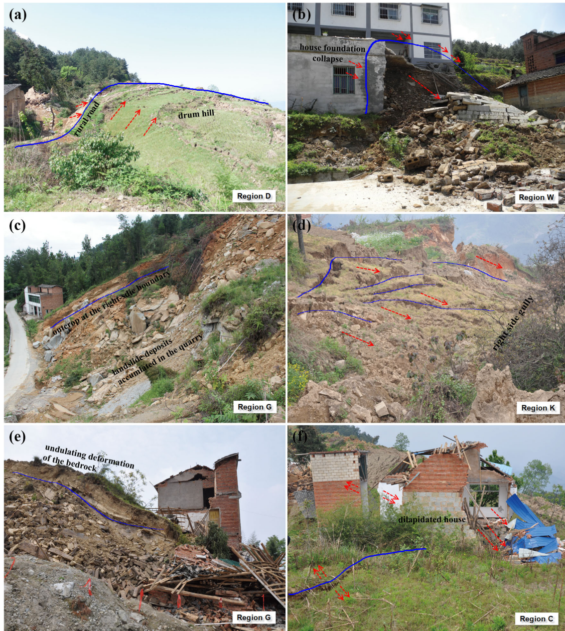
Fig. 8 Photographs taken by the authors showing the landslide deformation characteristics. a The drum mound formed by the landslide's extrusion in region D. b The house foundation that collapsed due to the bedrock collision in region W. c Landslide deposits in the quarry. d Slope deformation in region K. e Undulating deformation of the shale rock at the left-side of the landslide toe in region G. f Dilapidated houses in the upper part of the slide in region C. The locations of the photos taken are marked in Fig. 9
