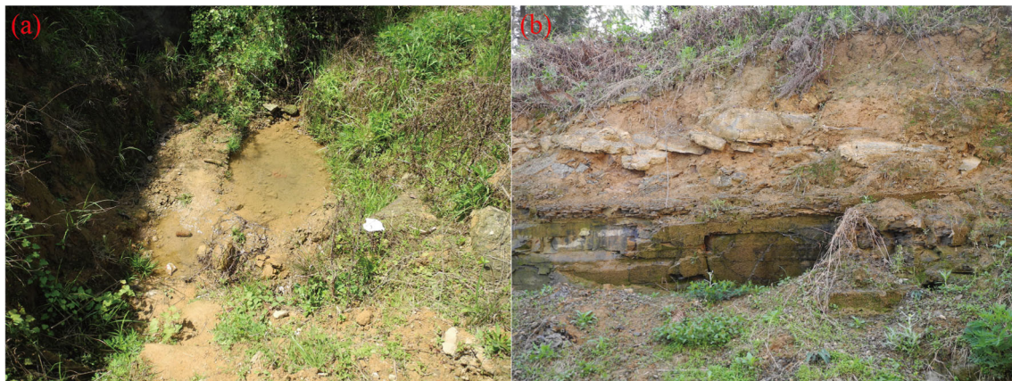
Fig. 4 Photographs taken by the authors showing. a Water spring at the back margin of the landslide. b Water seepage at the slope toe (see Fig. 2 for the locations of the photo taken)
