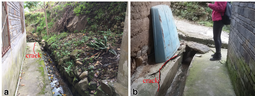
Fig. 14 Damage of drainage ditch. a The tension crack of drainage ditch and b the dislocation near the furrow bank
