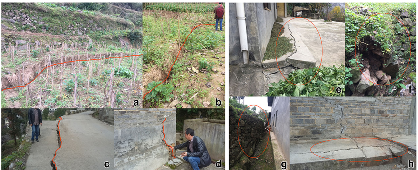
Fig. 4 Cracks and bulges have been observed within the landslide body. a Crack C1. b Crack C2. c Crack C5. d Crack C9. The locations of bulges are shown in Fig. 3
